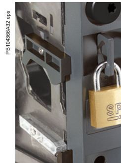
"Disconnected" position locking by padlocks.
